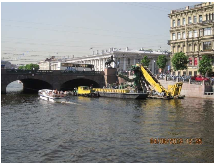
Work on clearing the bed of the river of Fontanka river section from Scherbakov lane to bridge Belinsky. 2013
